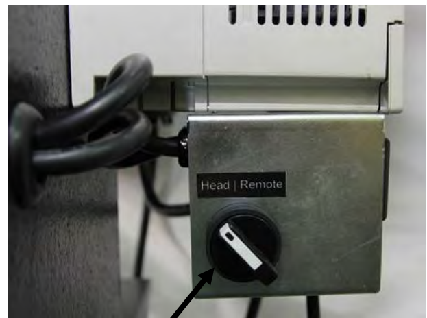
Controller selection switch
