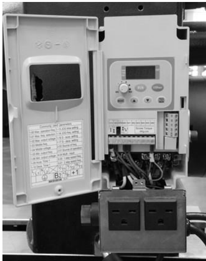
VFD with cover open
